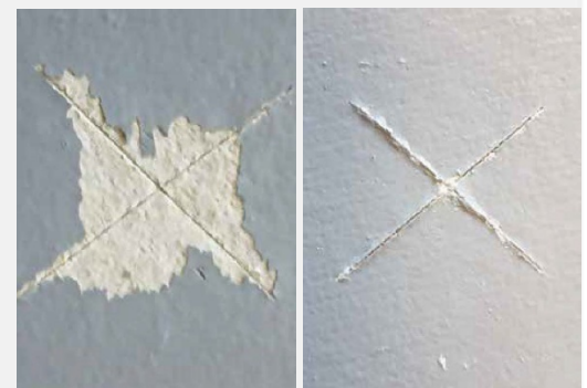
A simple cross hatch adhesion test reveals poor adhesion
