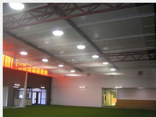
West Tamar Community Centre Training Facility's internal steelwork is primed with Durepon P14
