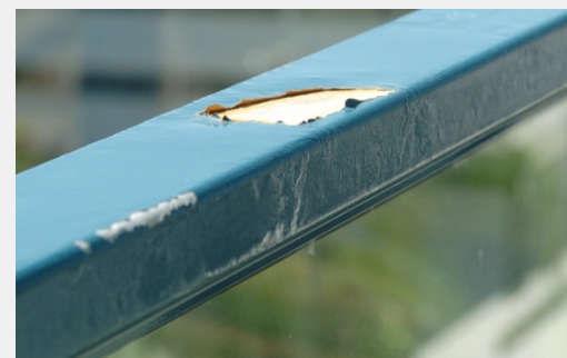
Inadequate coating thickness and humidity cause osmotic blistering
