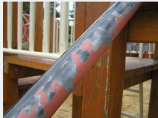
Underside of coating appears very smooth – little or no abrasion of the surface prior to painting
