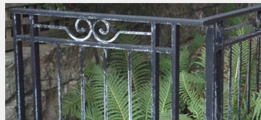
White rust appears on a micaceous iron oxide coating near a beachside residence.
