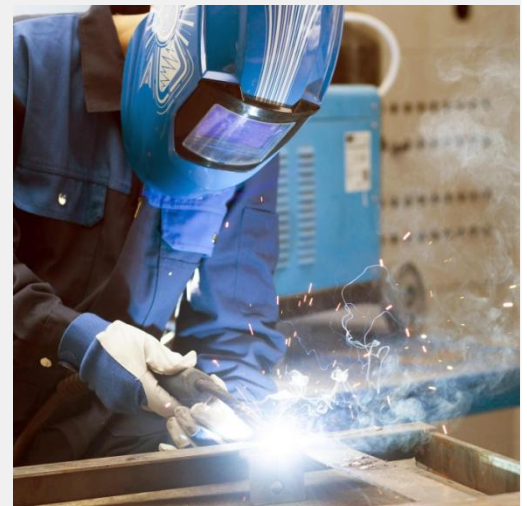
Heat from welding and grinding vaporises coatings and may be hazardous to inhale
