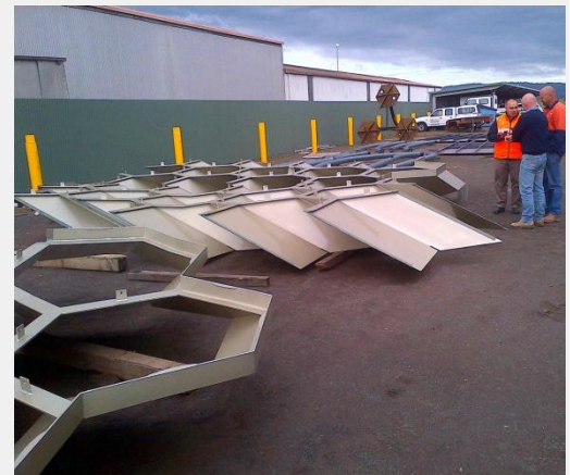
Federation Square Canopy was entirely prepared and painted in shop with Quantum ® FX, then welded together on site
