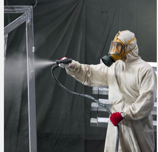
Spot priming and painting the cleaned welds and overlapping surrounding sound coating ensures continuous protection
