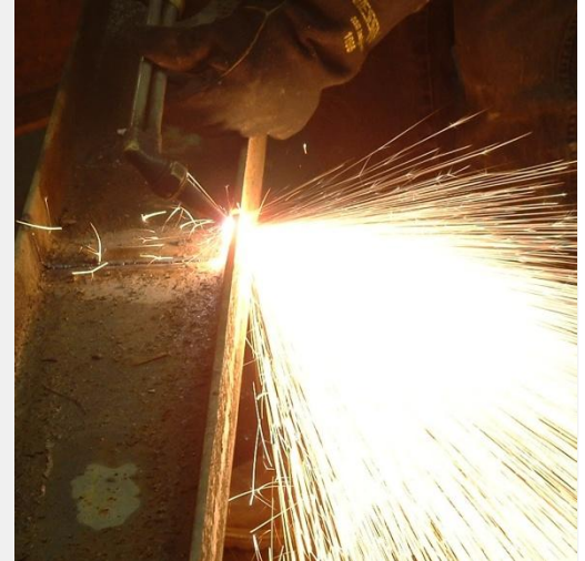
Both welding and grinding produce sparks that are hazardous to eyes and skin
