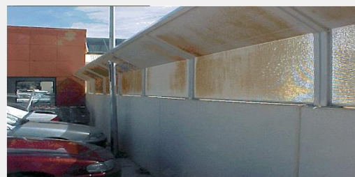
Screens in a two-year old bayside car park
