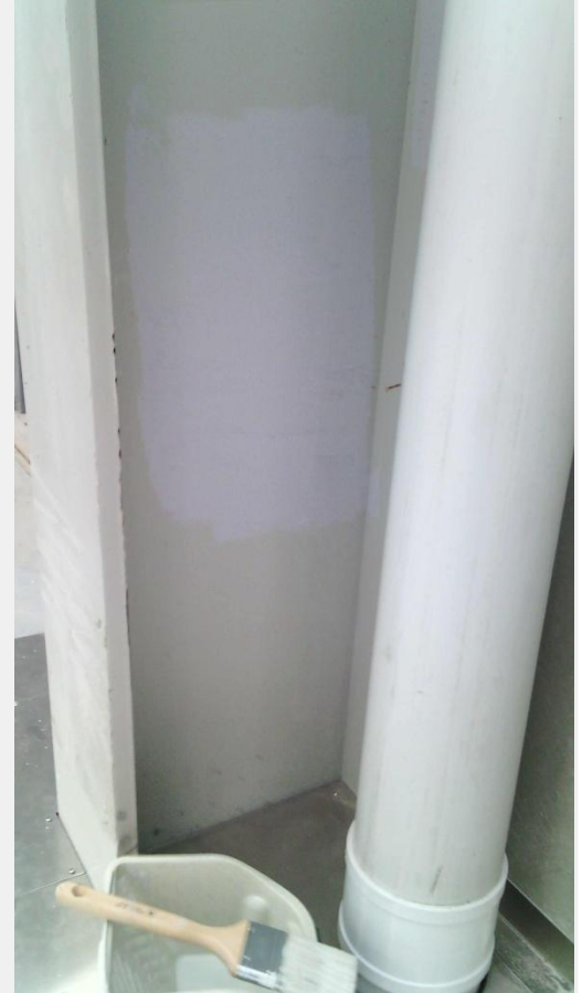
Freshly mixed zinc phosphate epoxy primer was applied over the same product applied only a couple of weeks earlier. Yellowing is clearly visible. As mentioned in the product's data sheet, this yellowing is expected, but will not detract from the protective properties of the product.
