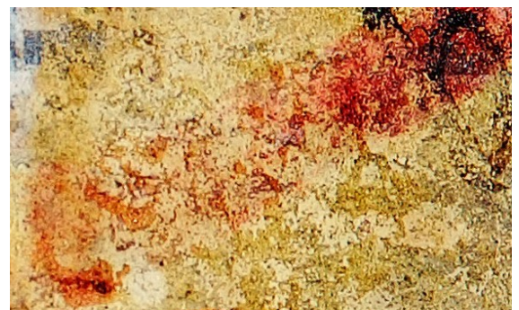
Red colour has penetrated and dyed the deteriorated, porous paintwork.
