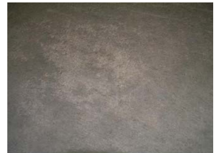
Laitance & roughness on concrete
