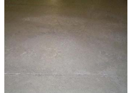
Laitance on concrete
