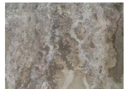
Efflorescence on concrete.
