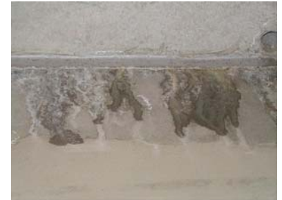
Efflorescence on concrete floor
